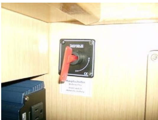
House battery switch
