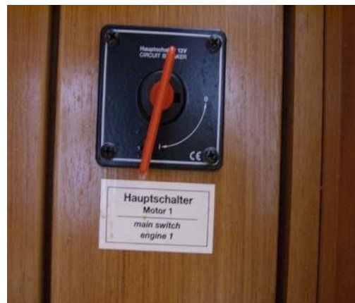
Engine battery switch
